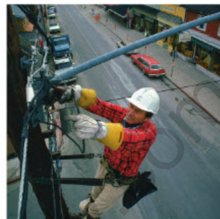
▲ People who work with electricity must be careful to use gloves made of nonconducting materials. Rubber, an excellent insulator, is often used for this purpose.
