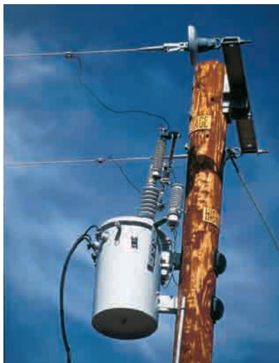
Figure 15.15 Electromagnetic induction in transformers delivers power efficiently and safely to your home.
