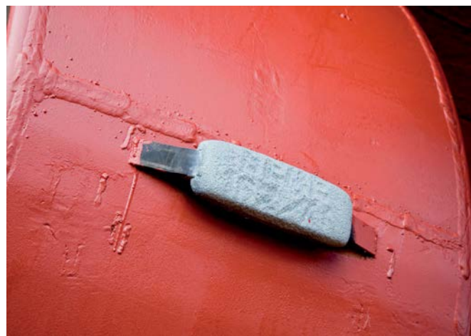
Figure 7.2 This is part of a ship's hull. It is made of iron protected by bars of magnesium metal. The magnesium atoms (oxidation number = 0) are oxidised to \text{Mg}^{2+} ions (oxidation number = +2) in preference to iron atoms changing to \text{Fe}^{3+} . This is called sacrificial protection.
