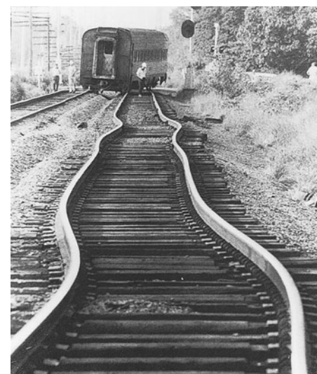
FIGURE 19-23 Railroad tracks in Asbury Park, New Jersey, distorted because of thermal expansion on a very hot July day.
