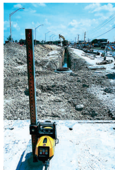
A laser-surveying instrument used to ensure proper placement of underground sewer pipes.
