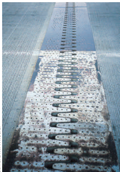
Expansion slots allow bridges to change length with temperature changes without damage.
