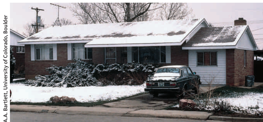
Figure 13-6 Melting snow patterns reveal differences in thermal conduction. For example, the old garage has been converted to living space, but it appears not to have been insulated.
