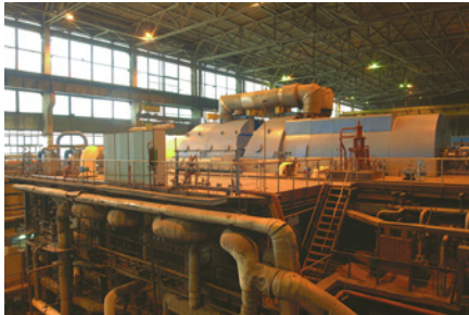
Figure 8.1 The same principles of electromagnetic induction apply in power stations but the scale is much bigger. The generator shown in Figure 8.1 can deliver 200 MW of power.
