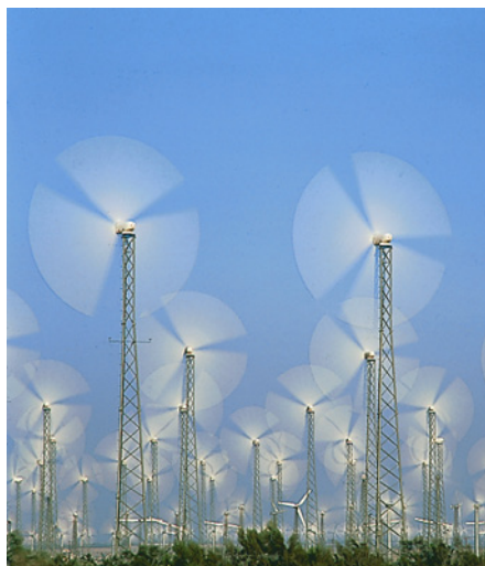
Figure 9.4 A large wind farm. Each wind turbine has three blades and can produce a power of up to 3 megawatts. Such a large farm can be equivalent to a coal-fired power station.
