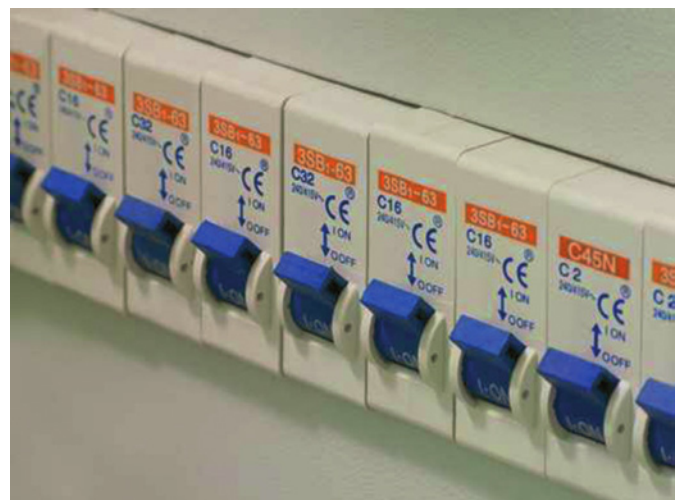
Figure 2.8 Circuit breakers in a modern fuse box.
