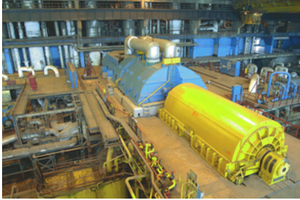
Figure 8.3 This shows several 600 megawatt generators inside the coal-fired Drax power station. Superheated steam is used to drive the generators.
