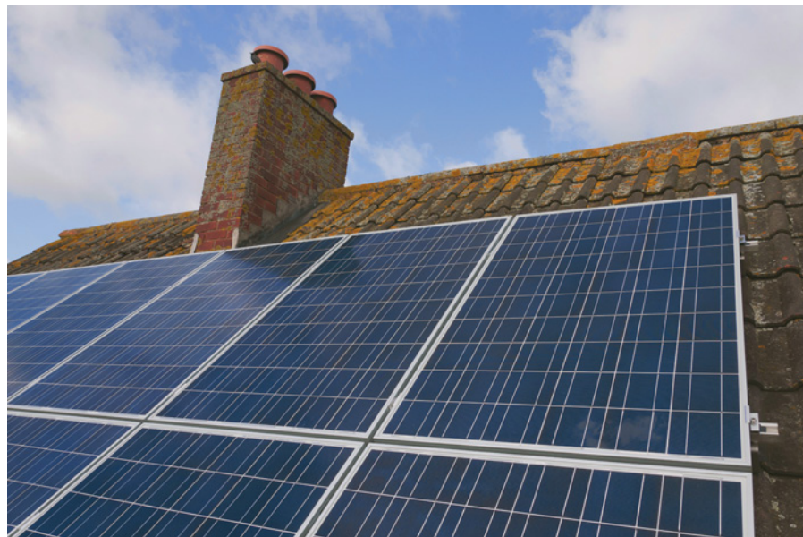
Figure 4.3 Solar panels in this house provide the householder with electrical energy. The blackened surface allows infra-red radiation to be absorbed efficiently.
